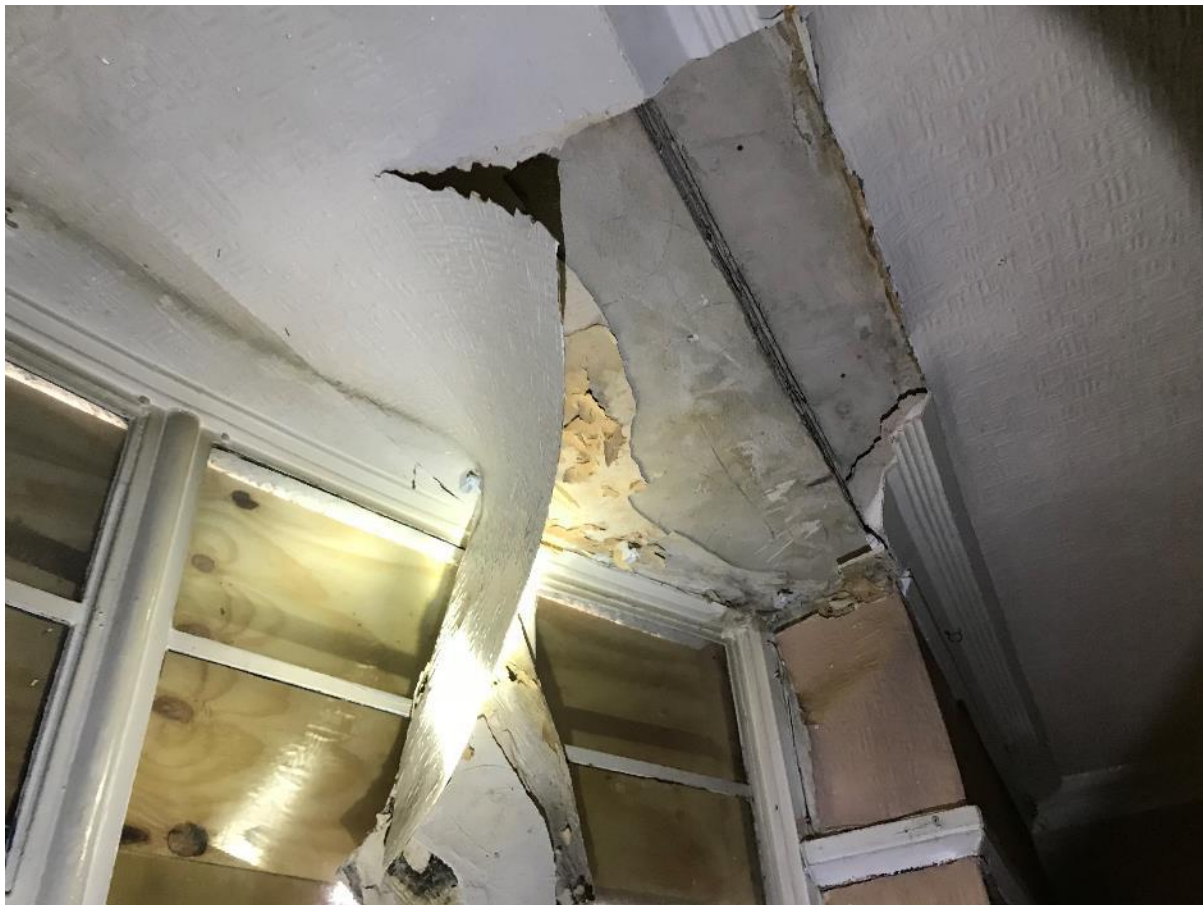
Roof leak / collapsing ceilings
